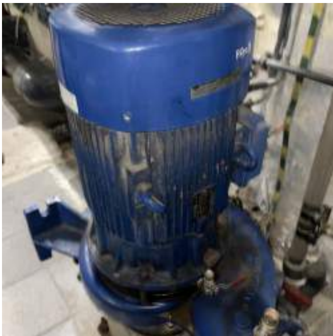
Figure 20 Water circulation pump for the pool water treatment system
