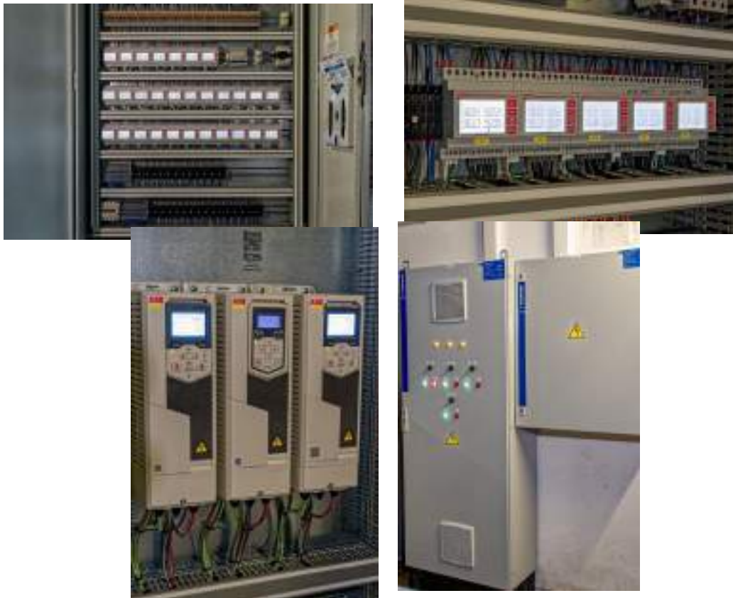
Figure 16 Panels after the energy meters and inverters
