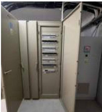
Figure 17 Existing main electrical switchboard
